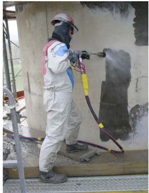
2 x 2500 bar operating pressure to free 2000m 2 steel reinforced concrete walls from top layers
